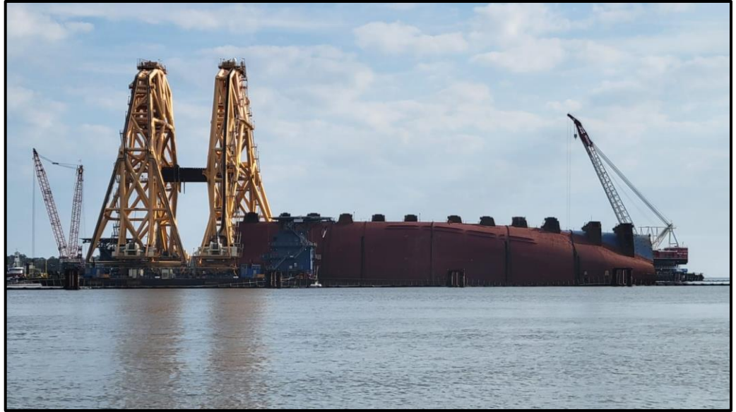
Photo: The VB-10000 moved off Section Seven to prepare for cutting operations on Section Two on Saturday. St. Simons Sound Incident response photo
