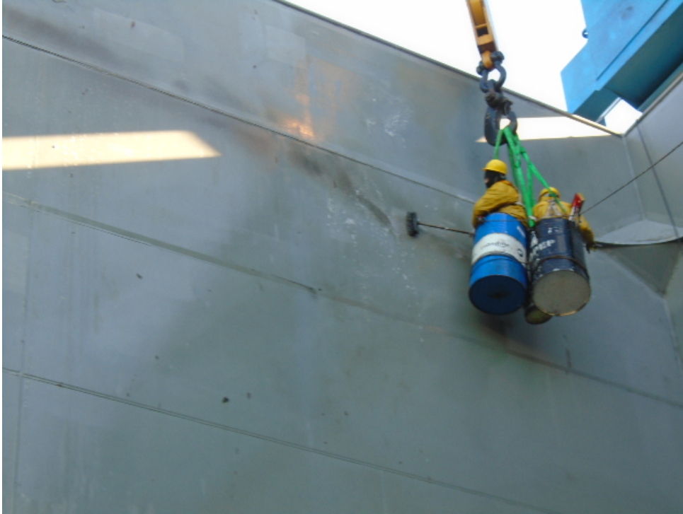
Ship's crew cleaning the Bulkhead at remote anchorage with Aqua Tuff after discharging Coal
