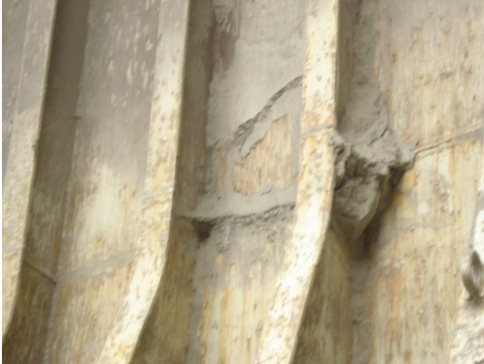
Cement became solid and hard in between the frames
