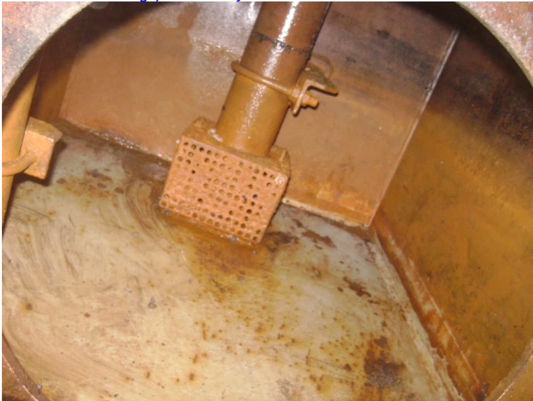
Condition of Hold Bilge, Clean & Dry
